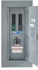
NQ MB Panelboard with SurgeLoc SPD installed
